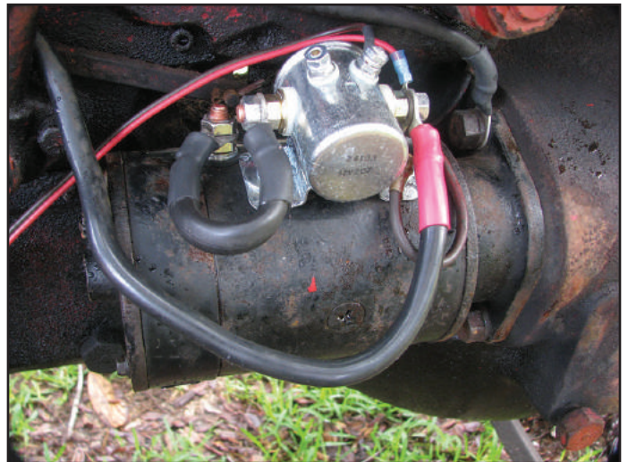
Figure 6 – A starter solenoid was mounted on the starter's to replace the mechanical switch.
