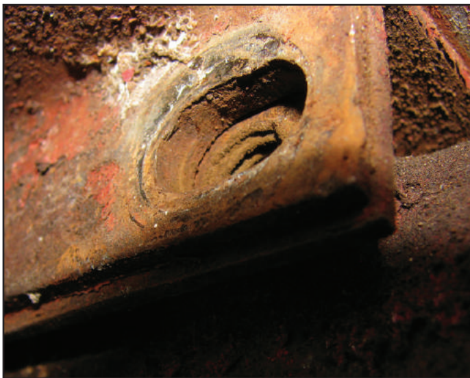
Figure 4 – Once the ground cable bolt was removed, the condition of that electrical connection became obvious.
